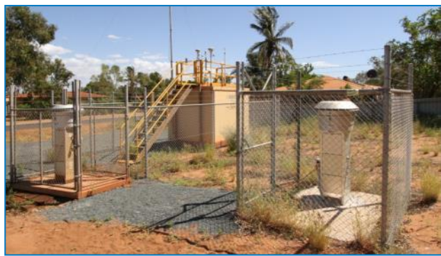
Figure 2-3: Taplin Street Monitoring Station
