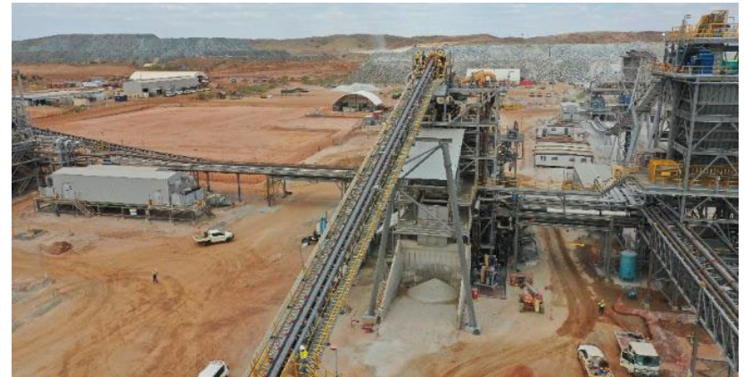
Primary Rejection Infrastructure October 2023
